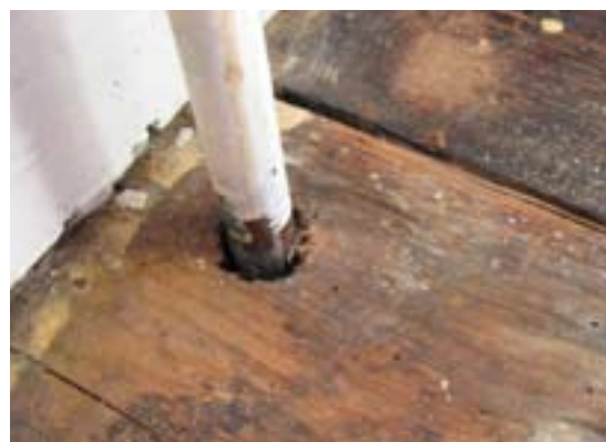
Figure 5 Air leakage through gaps around service pipes in suspended timber floors
