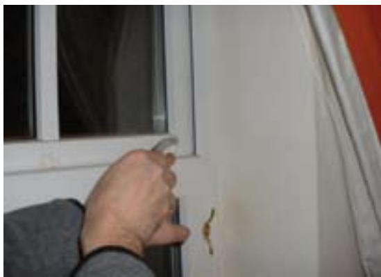
Figure 7 Air leakage around opening window casements
