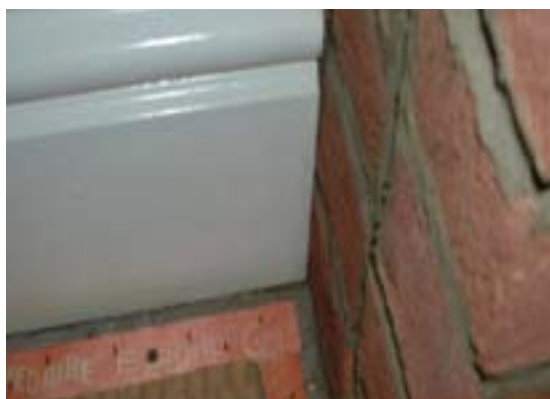
Figure 3 Air leakage path hidden behind skirting board
