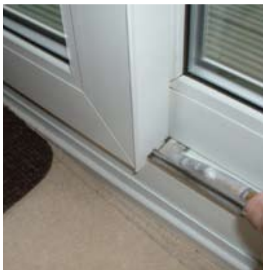
Figure 9 Air leakage around the slide mechanism of patio doors
