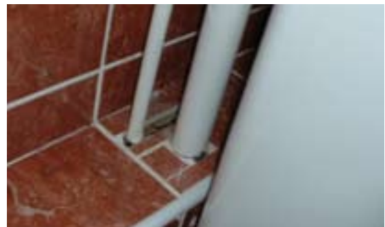
Figure 15 Draughts may be felt around bathroom sinks and vanity units
