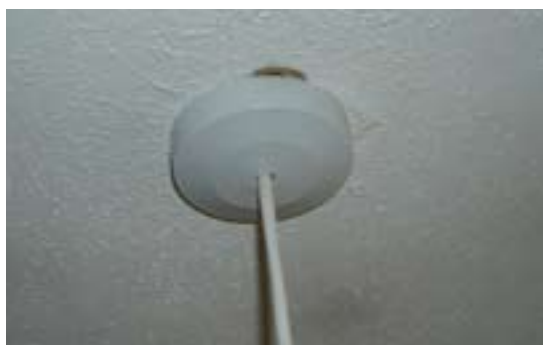
Figure 10 Air can leak through gaps around light fittings into the roof void
